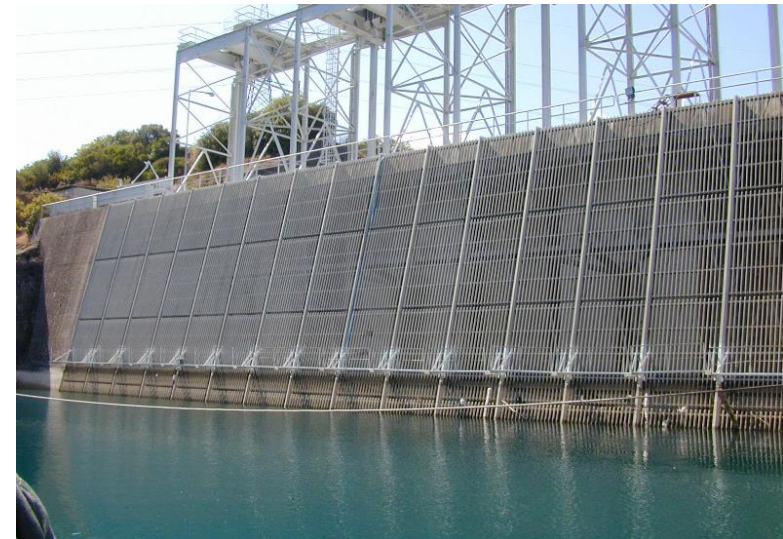
Kastraki dam: trash racks and gates
